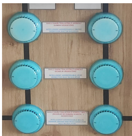
Smoke and Heat Detectors
